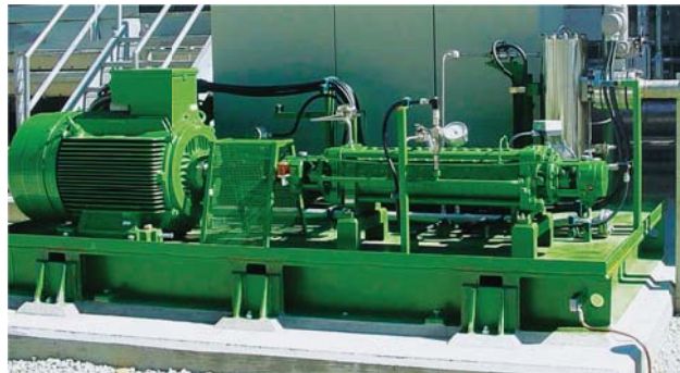
Figure 2-8: Typical wet compression demin pump skid with VFD
