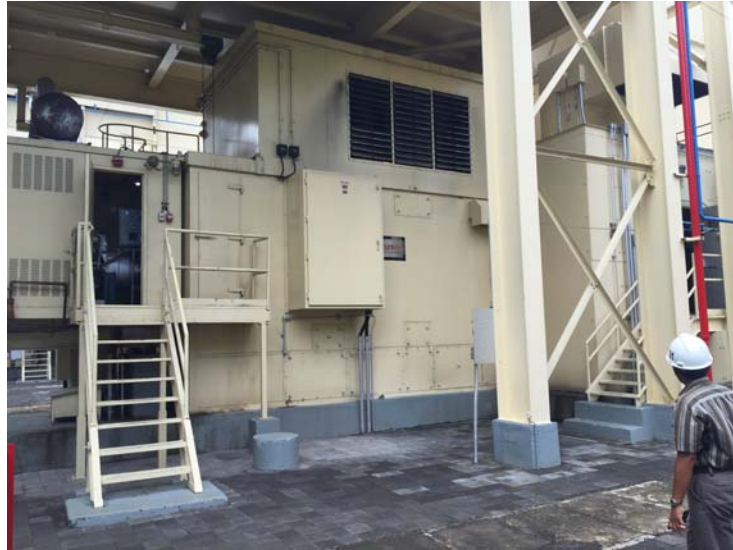
Figure 3-3: Pesanggaran Unit 3& 4 (typical)
